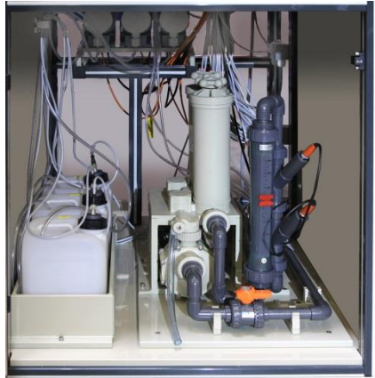
Inside view of the PRS with reservoirs for electrolyte stabilization and pH regulation, dosing pumps, circulation pump M50, filter cartridge unit 2 x 10", flow meter and flow adjustment valve
