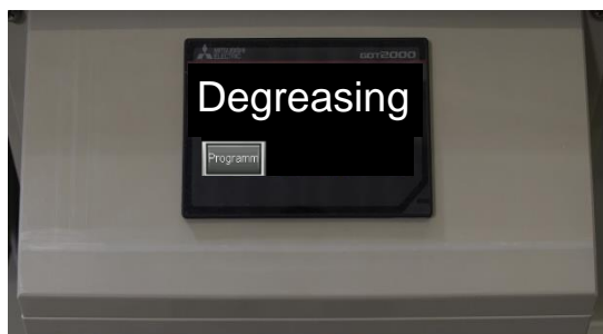
Control panel for process control (Example: degreasing)
