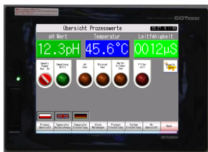
Adjustment and monitoring of the bath parameters by the Touch screen operators' terminal (PRS control)
