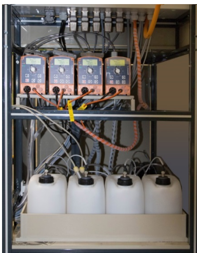
Inn view of PRS: Dosing pumps and reservoirs for regulation chemicals for plating bath
