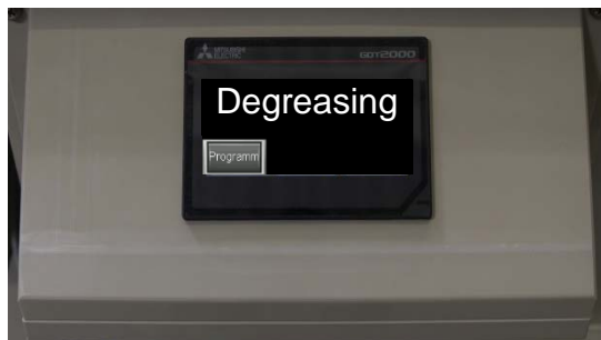
Control panel for process control (Example: degreasing)
