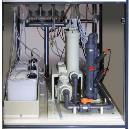
Inside view of the PRS with reservoirs for electrolyte stabilization and pH regulation, dosing pumps, circulation pump M50, filter cartridge unit 2 x 10", flow meter and flow adjustment valve
