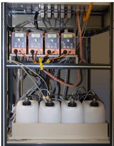
Inner view of PRS: Dosing pumps and reservoirs for regulation chemicals for plating bath
