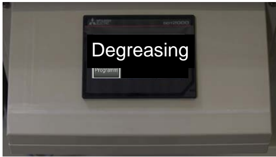
Control panel for process control (Example: degreasing) 控制操作程序的触控板 举例：去脂
