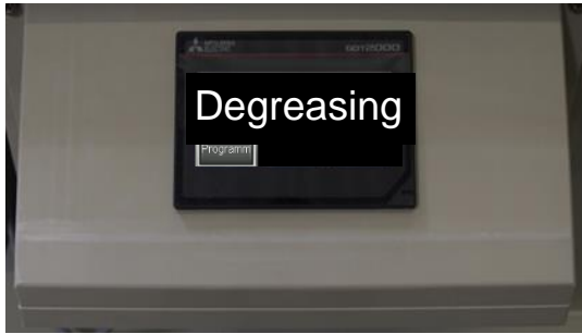
Control panel for process control (Example: degreasing) 控制操作程序的触控板 举例：去脂
