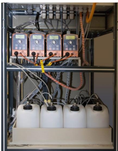
PRS 内视图：计量泵和镀槽化学剂的贮池 Inner view of PRS: Dosing pumps and reservoirs for regulation chemicals for plating bath
